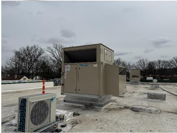
ECC – Roof Top Units Install In Progress
